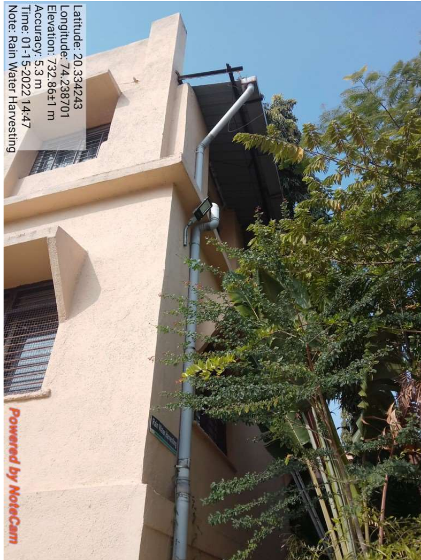
Figure 2. Rain Water Harvesting from Roof top of the buildings
